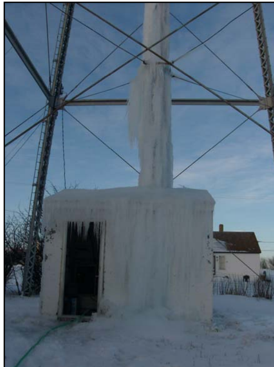
The City of Flaxville used a Renewable Resource Emergency grant to repair the town water storage facility Tank February 2014
