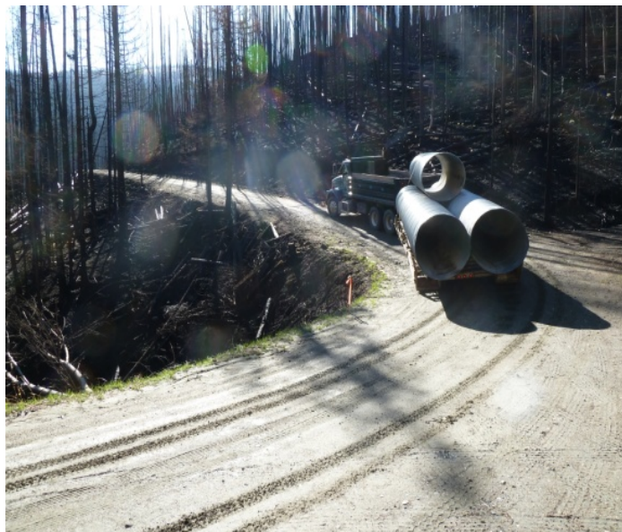
Figure 3. Large culverts being installed within areas burned by the Saddle Fire to protect Beaver Creek Road (Forest road 91) from washing out (photo taken 10-14-11).
