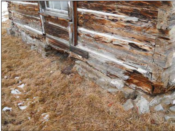
Figure 23: Failing foundations and rotting logs need to be addressed
