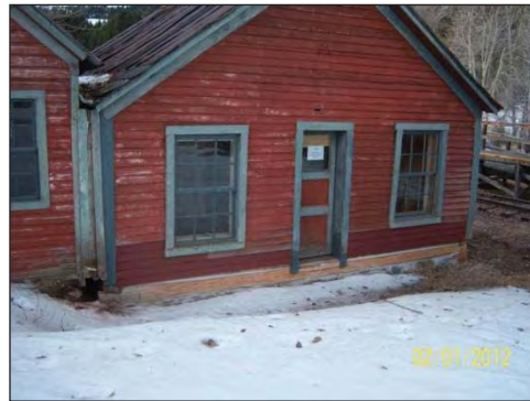
The “Restaurant” on the right has been stabilized and sits well above grade
