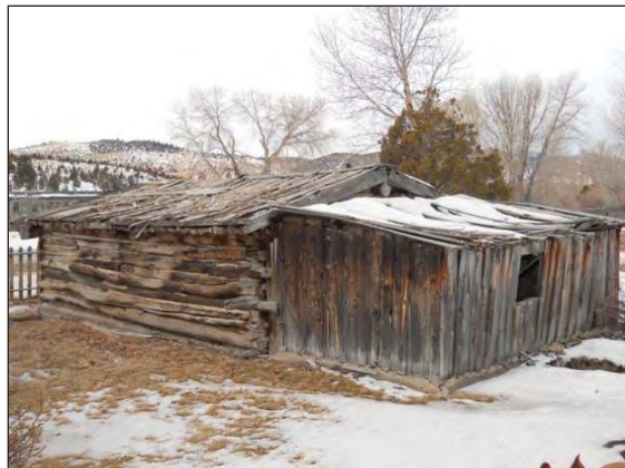
Figure 17: Rear portion of Richards Cabin collapsing- safety issue
