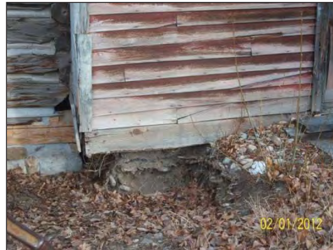
Non-preserved building has virtually no foundation and rotted sill logs
