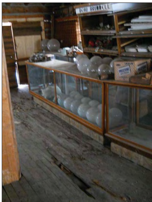
Figure 21: Charlie Bovey Building in desperate need of stabilization- floor is sunken in, endangering collections
