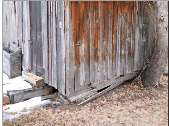
Figure 24: Iron Rod Cabin needs a foundation and weatherproofing
