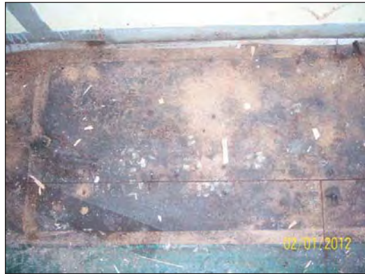
Water damage in the NR listed Dr. Don L. Byam house
