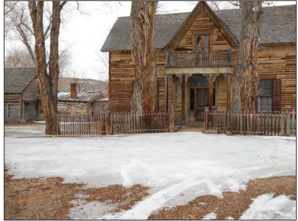
Figure 14: Poor drainage creates a sheet of ice in front of the Sedman House, an impressive structure that needs to be treated by painting
