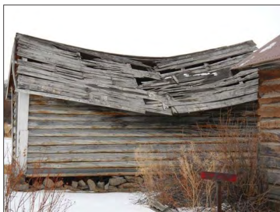
Figure 19: Collapsing roof is a safety issue
