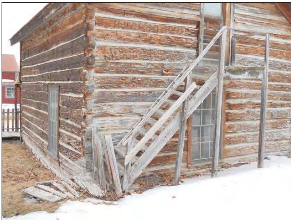
Figure 15: Rotting boards require consolidant
