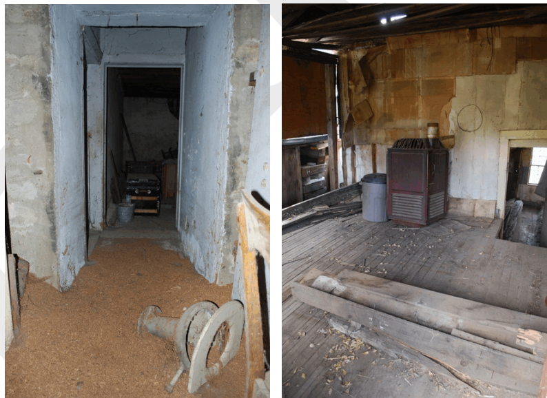
Examples of preservation work needed in Virginia City. Left, the back of the E.L.Smith Store. Right, Cogswell Cabin where the log wall on the left has rotted away. Photos by Hope Stockwell
