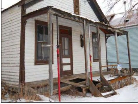
The rotted porch and failed stone foundation of the Hickman House
