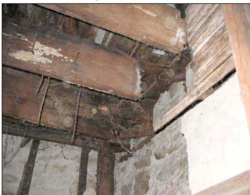
The E.L. Smith Store has structural issues both inside and out
