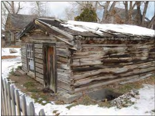
The Richards Cabin, an original structure, has major drainage issues
